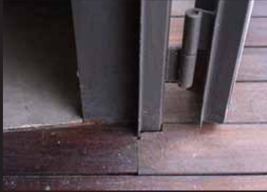
9-07_11_Hitches terrace door
