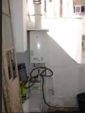
8-08_28_heater and counter
