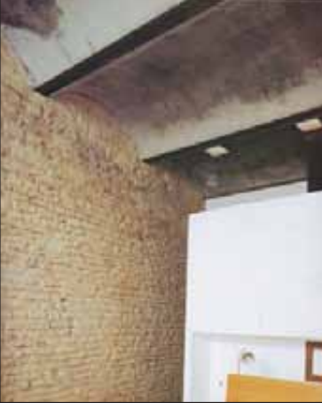
prefab concrete vaults /
